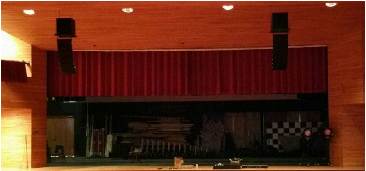
Example of Rigged and suspended speakers.
