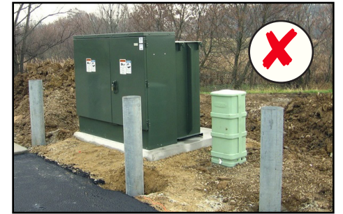
Utilities and service lines should be concealed.
